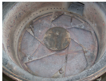
Fig. 3. View of combustion chamber with rotating grate
